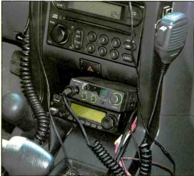
This is entitled “How Not to Do It!” This is the first installation I did when I got the truck. I needed 2 meters and CB fast so I just jammed them in and let the wires fall where they may. Ugly and cluttered are two words that jump immediately to mind. Too many wires in the way. We can do better.
